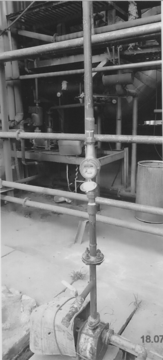
TREATED WATER FLOW METER
