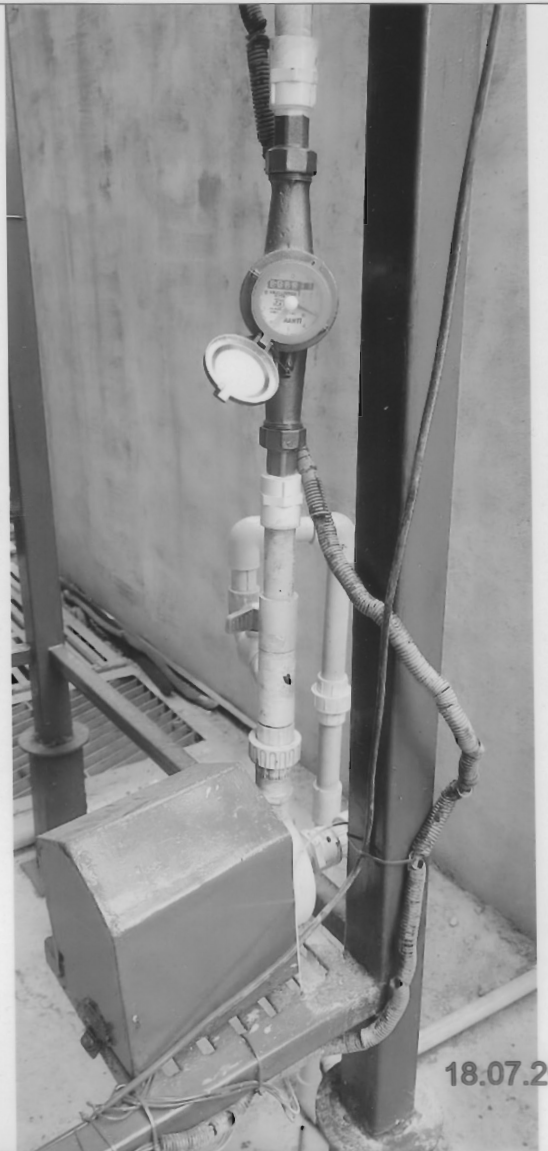
INLET FLOW METER
